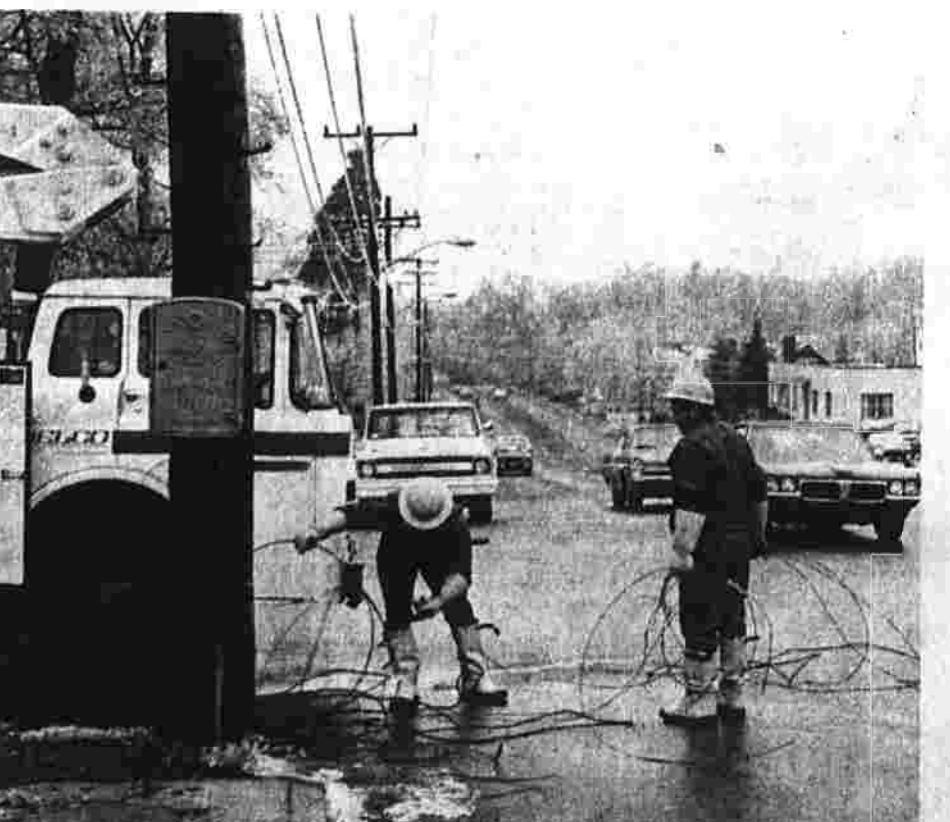
Big Task For Power Company Crews It was a short night and will be a long day for Hartford Electric Co. (HELCO) crews as they work to restore electric service to homes and business in the wake of a storm early today. The rain-turned-to-ice storm severed power lines throughout Manchester and in many other parts of the state. The first outage was reported about midnight and continued until early morning. (Herald photo by Buccevicus)
